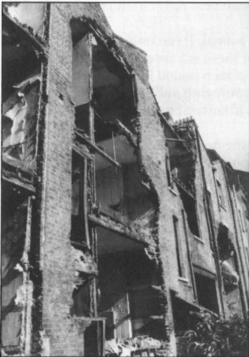
This destruction in 1984 of the rear walls was deliberate.
