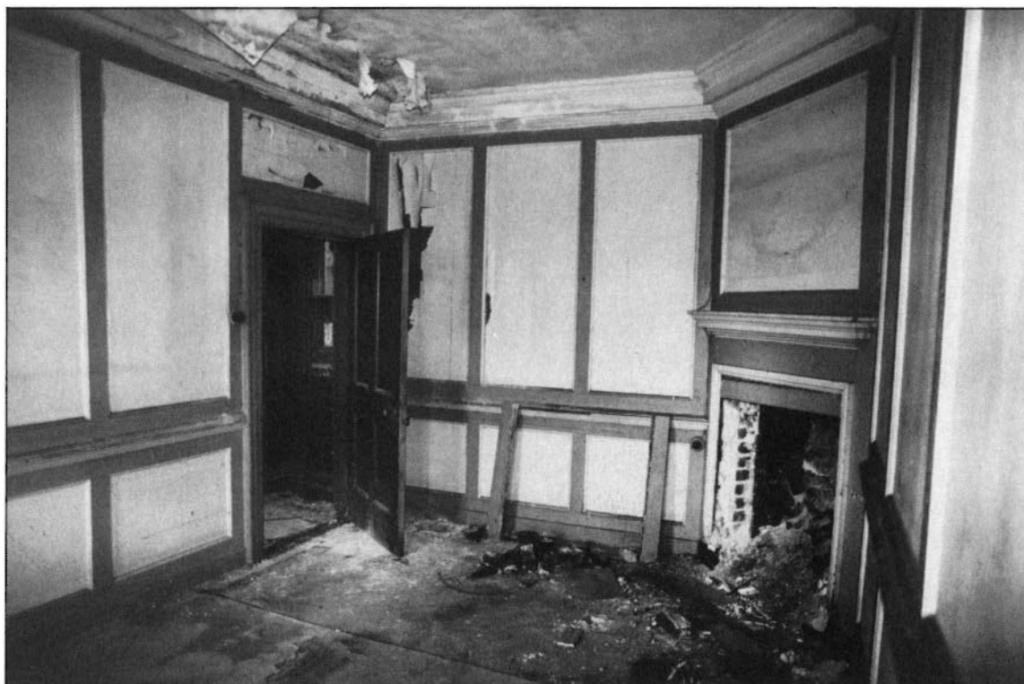
A rear room with timber panelling of c1740. This photograph was taken in 1983 since which time there has been a major water penetration.
