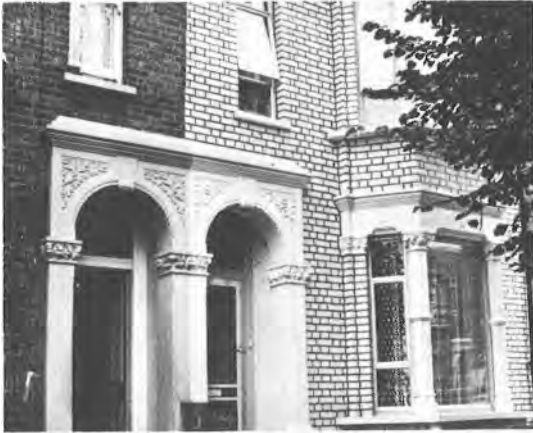
This newly painted house has an unreal cartoon-like character which stops dead at the junction between the two houses.
