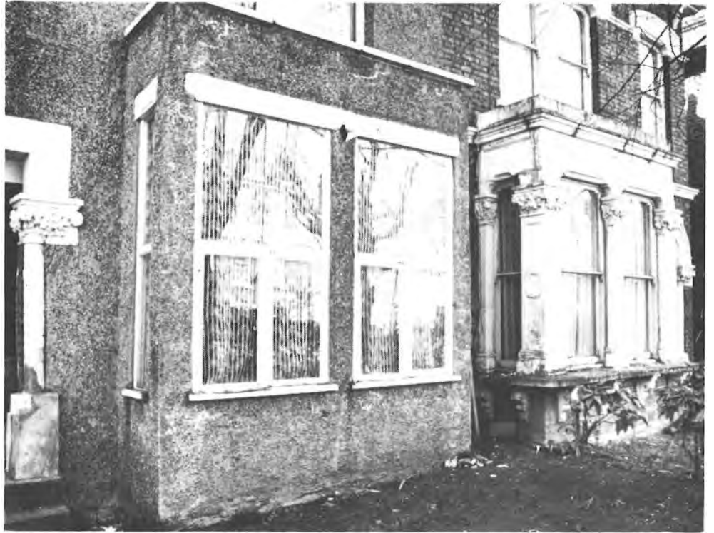
This new bay window has no advantage over the original; it gives no extra space or light and lacks character.
