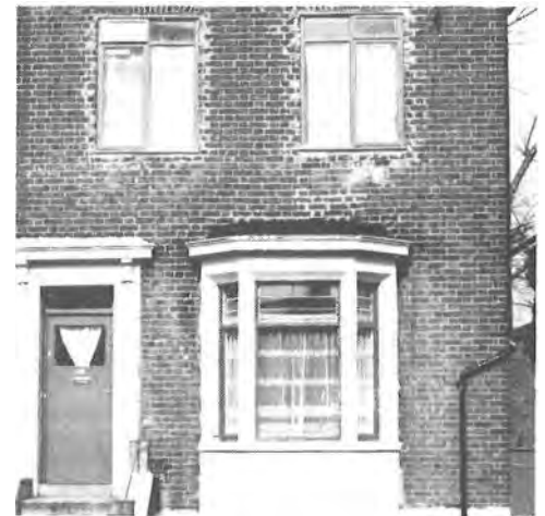
Patchy brickwork due to removal of original windows - new window size has no advantage over the old.
